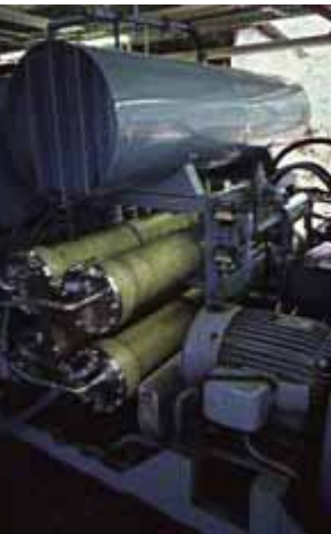
Reverse osmosis desalination unit in the Virgin Islands, United States
